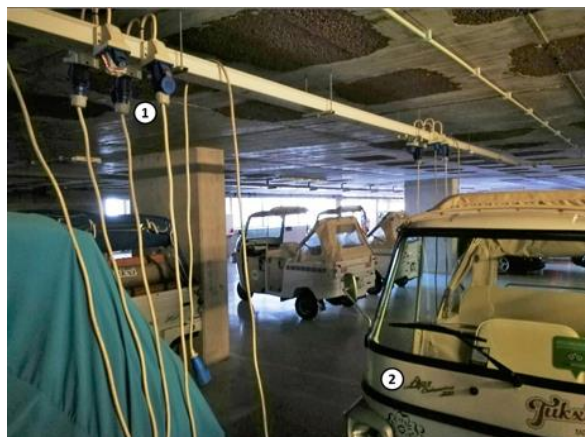
Figure 7.5 – Electric Vehicle charging infrastructure in the Tukxi Eco Tours facilities. The number 1 represents the 16 A sockets user for charging, and the number 2 shows one of the electric vehicles being charged.
